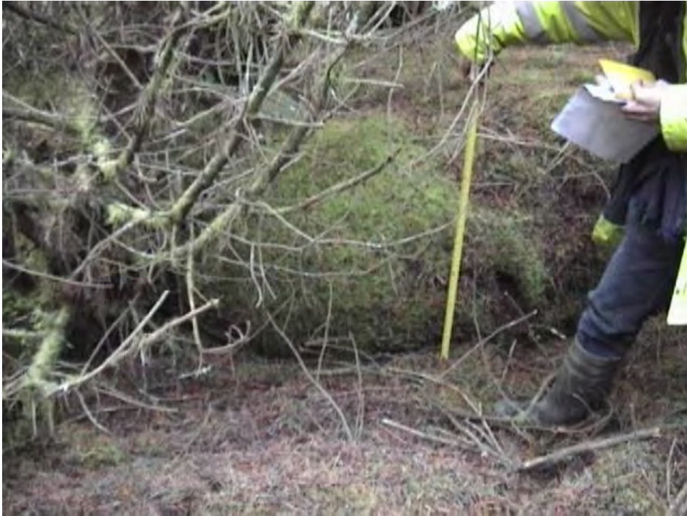
T29 – Bearing Failure South of Access Road and Arisings.
