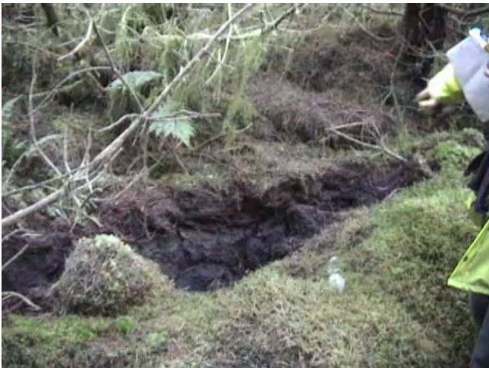
T29 – Tension Crack at Tree Line
