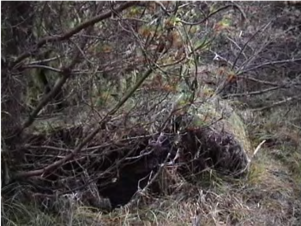
T66 – Bearing Failure South of Access Road and Arisings.
