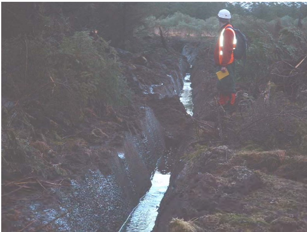
T14 – Collapsed Drain.
