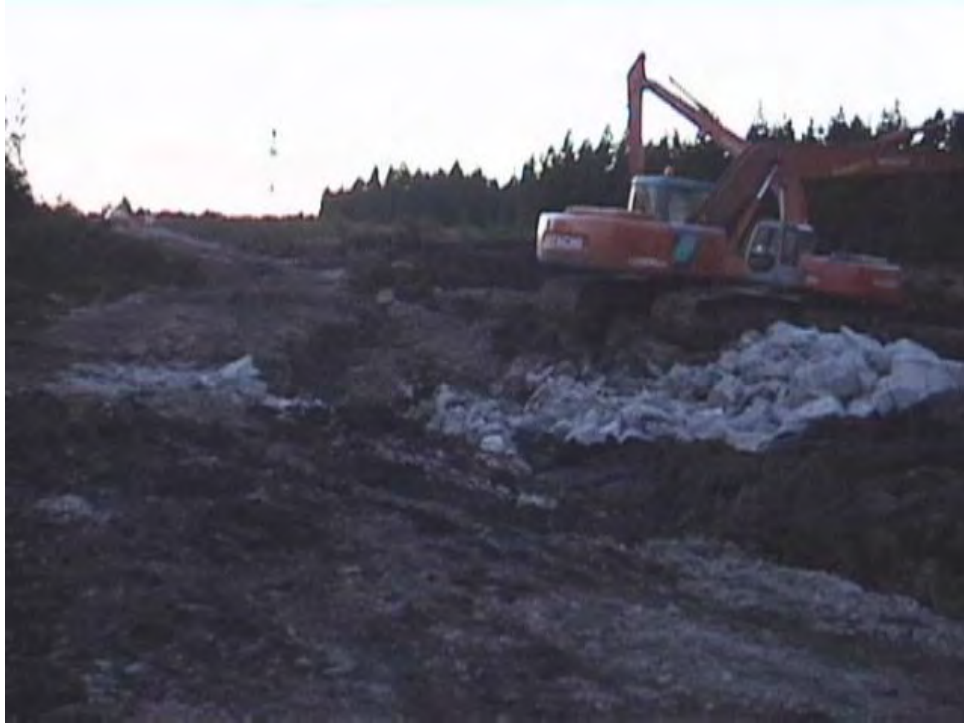
T68 – Crest of Failure, Bowing of Access Road.
